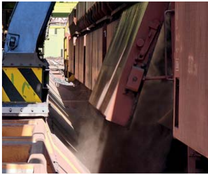
Figure 2. Suction system at the side of the wagon
